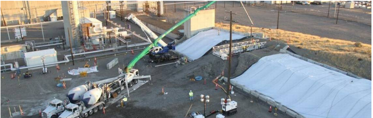
Grouting operation in November, 2017 to stabilize the smaller PUREX tunnel after a section collapsed.
