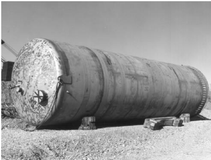
An unused steel cylindrical tank is shown prior to its insertion into a concrete silo. Fill pipes will be attached to the top of the tank while its base will be anchored to the floor of the concrete silo.
