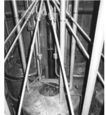
The interior view of a large concrete silo illustrates the complex system of pipes used to fill each of the four to seven cylindrical tanks within each silo.
