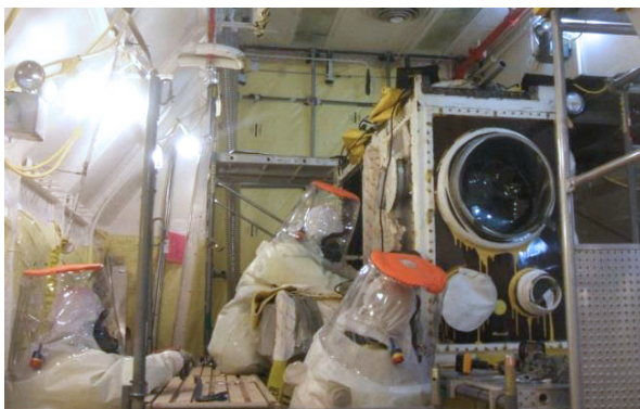
Sealing of one of the large 12' gloveboxes at the Hanford Plutonium Finishing Plant (PFP) in February, 2016.
