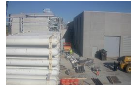
Zucrow High Speed Propulsion Lab
