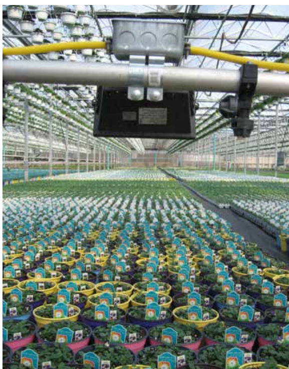
Figure 6. This boom-mounted high-intensity lamp operates during the night to provide intermittent light to the crops below.
