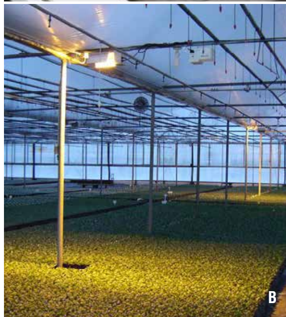
Figure 7. High-pressure sodium lamps with oscillating reflectors (A) cast moving beams of light to crops below (B).
