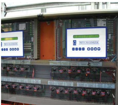
Figure 1. Some units will accept 30 or more sensors and control 40 or more stages.
