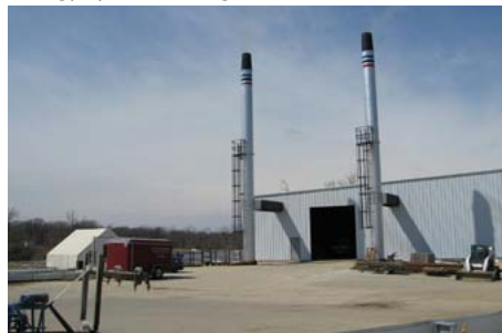
Fig. 1 Wood Burning Furnaces for Heating Greenhouses
