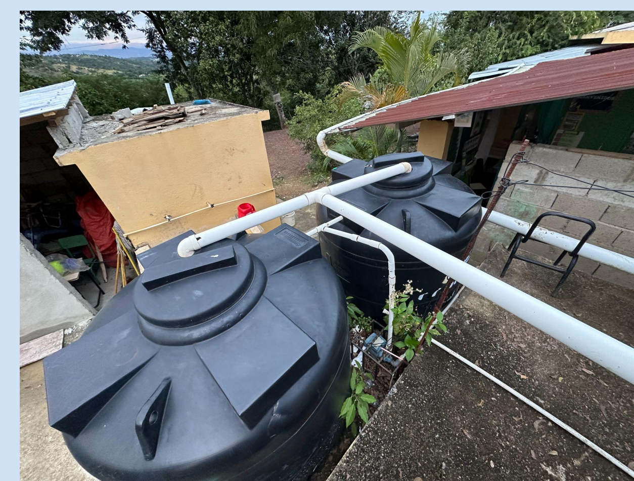
May, T. (2023) Rainwater collection system at Desecho Education Center
