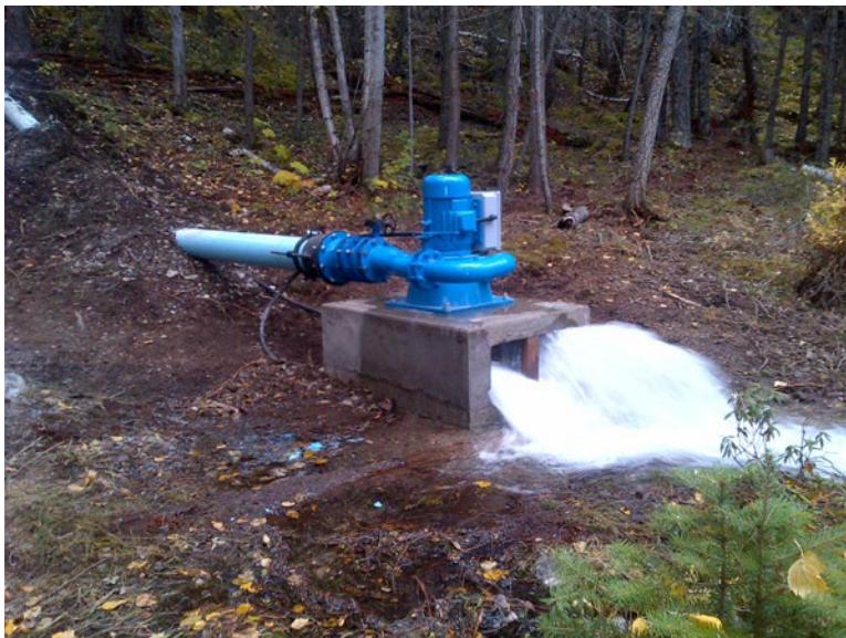
Figure 7-4: Micro hydropower facility (Source: Suneco Green Energy [8])
