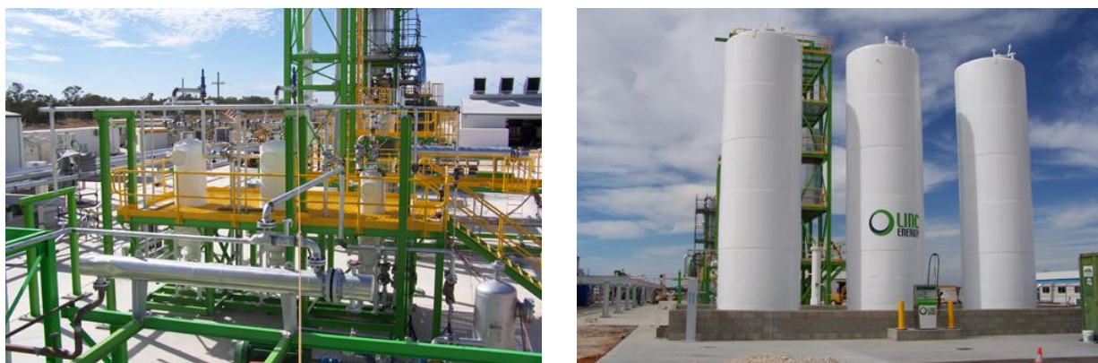
Figure 6. Chinchilla site image - GTL pilot plant commissioning, May 2008 ( http://www.lincenergy.com.au ).
