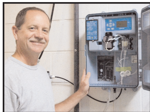
Gary Rossetter, Water/Waste Water Operator, installs an analyzer that will monitor the water 24 hours a day to help improve Purdue's water quality.
