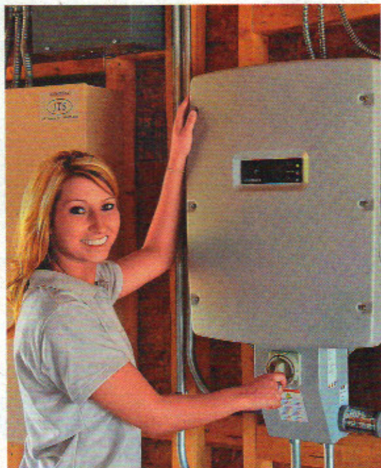
McKenna J. Regan, a member of the Purdue Solar Decathlon team, stands next to the solar house service panel.
