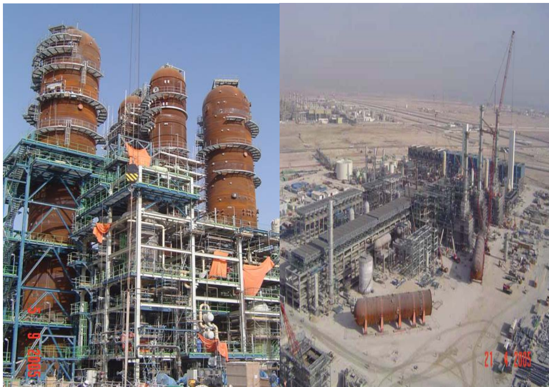
Figure D.15. Construction of the SASOL Oryx Plant in Ras Laffan, Qatar
