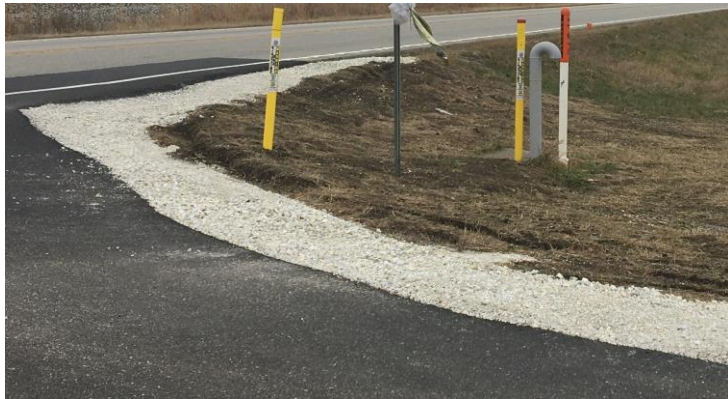
A filled and compacted stone shoulder is a low cost way to prevent crashes.
