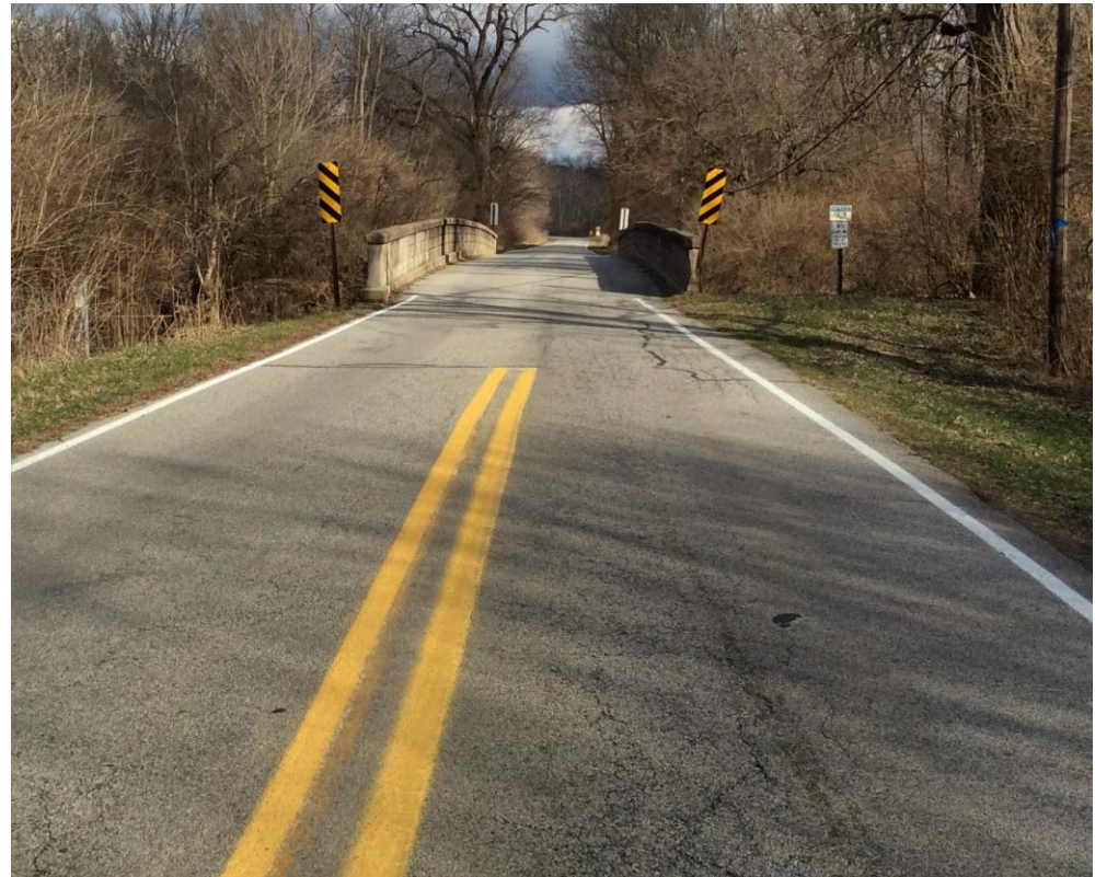
A warning sign is needed on each approach for this narrow, one-lane bridge.
