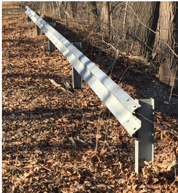
This guardrail is a potential hazard since it has no end treatments.
