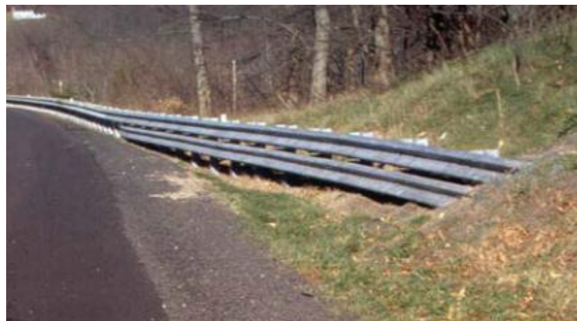
This is the safest way to bury guardrail ends. Picture courtesy of WSDOT.
