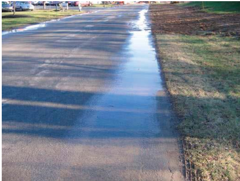
Left untreated, this ponding water will eventually damage the pavement.
