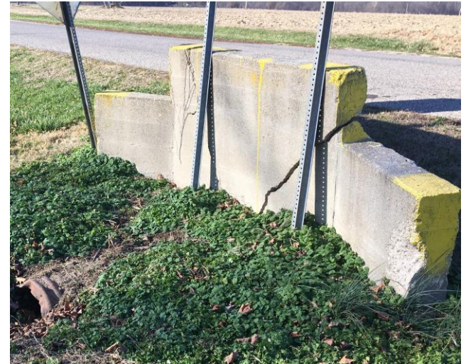
This old headwall is presents a potential hazard to motorists and should be replaced with a safer design.
