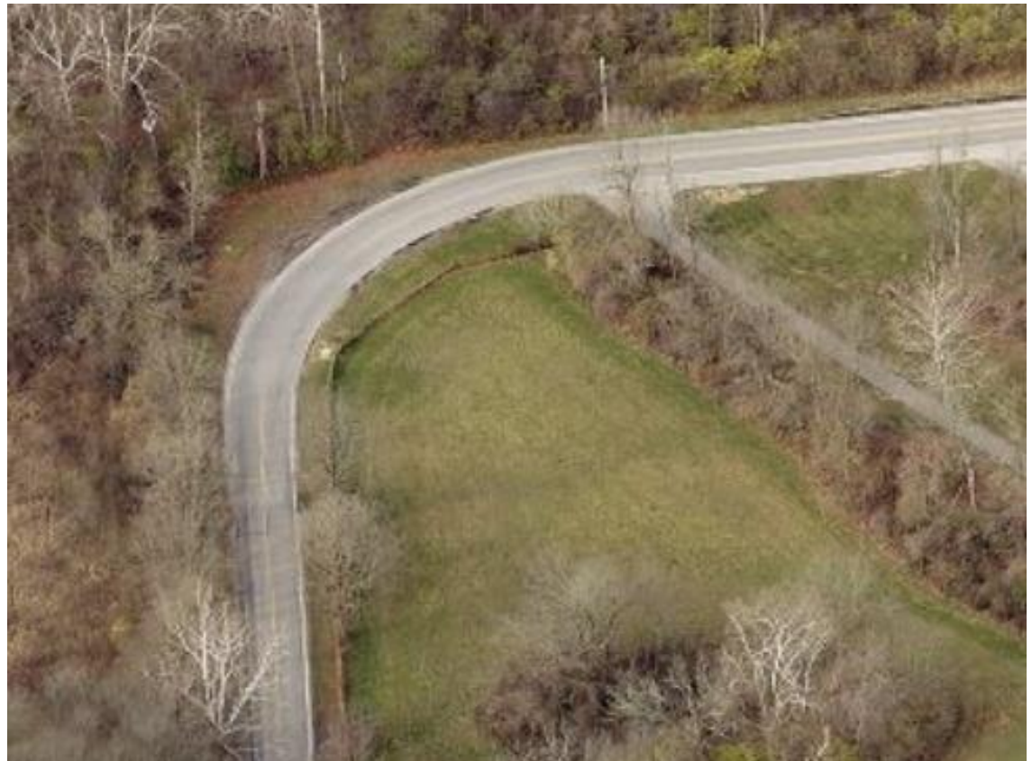
Boone County cleared back outside of this curve to provide a forgiving roadside, in addition to fixing pavement issues that were causing drivers to lose control at that curve.
